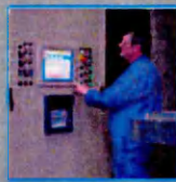
SPF Control System
